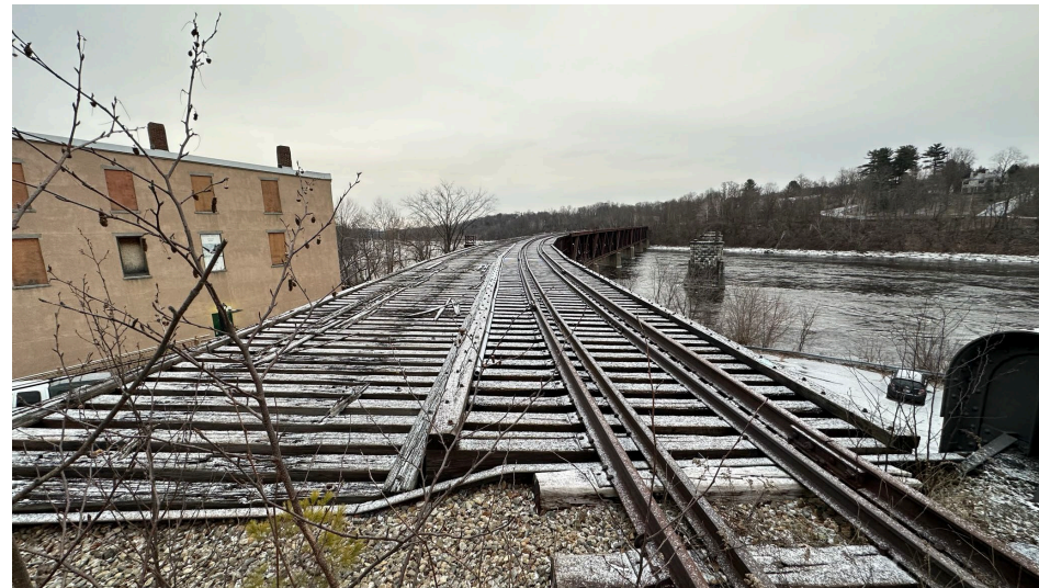
Kennebec River Bridge – Augusta (OOS - 1 Track Removed)
